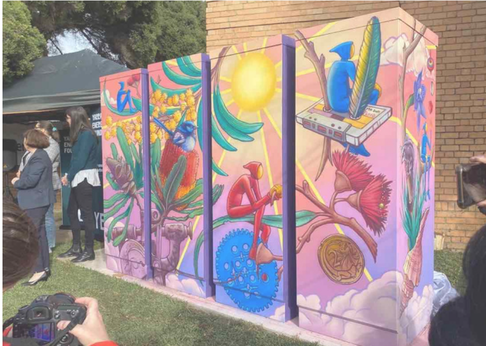
Community Battery installed in Fitzroy, image by Brant Kozlovskis, Pixii, LinkedIn
