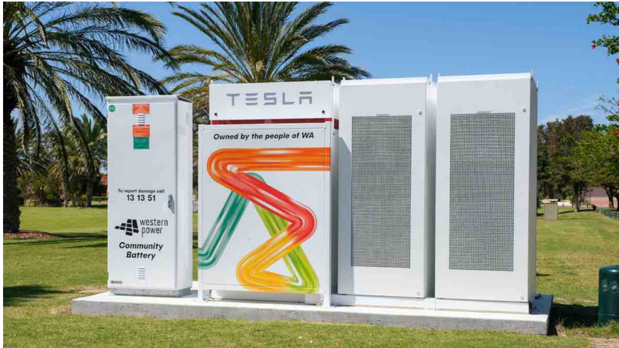
Image of the community battery installed as part of a W.A. trial.
