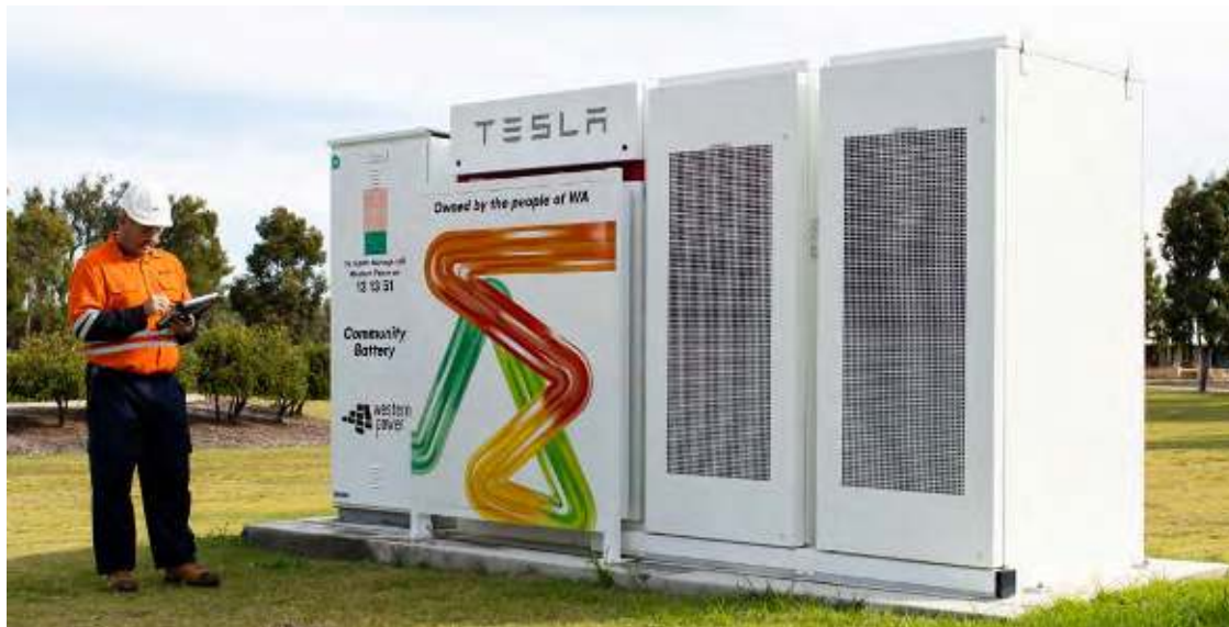
Image 1. Western Power PowerBank Battery Source: DELWP Victorian NBI Consultation Paper
