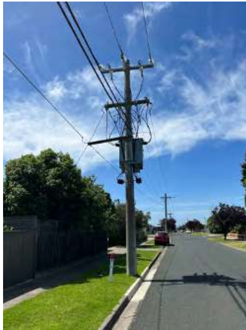
Image 9. Typical Powercor Pole mounted transformer in the Geelong Region
