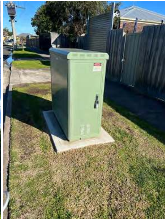
Image 14. LV Distribution Switchboard
